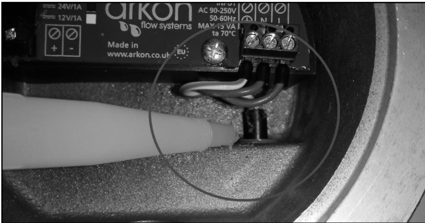
Pic. 2 Application of silicon binder on cable sheath of opened round cross cut cable end
